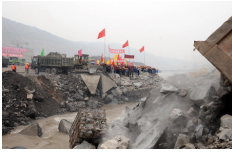
Workers empty out trucks loaded with rocks and stones to block the Jinsha River at Xiangjiaba, southwest China. The third largest hydropower plant in China, which is expected to be completed by 2015, will be able to generate 30.7 billion kw hours of electricity a year.
